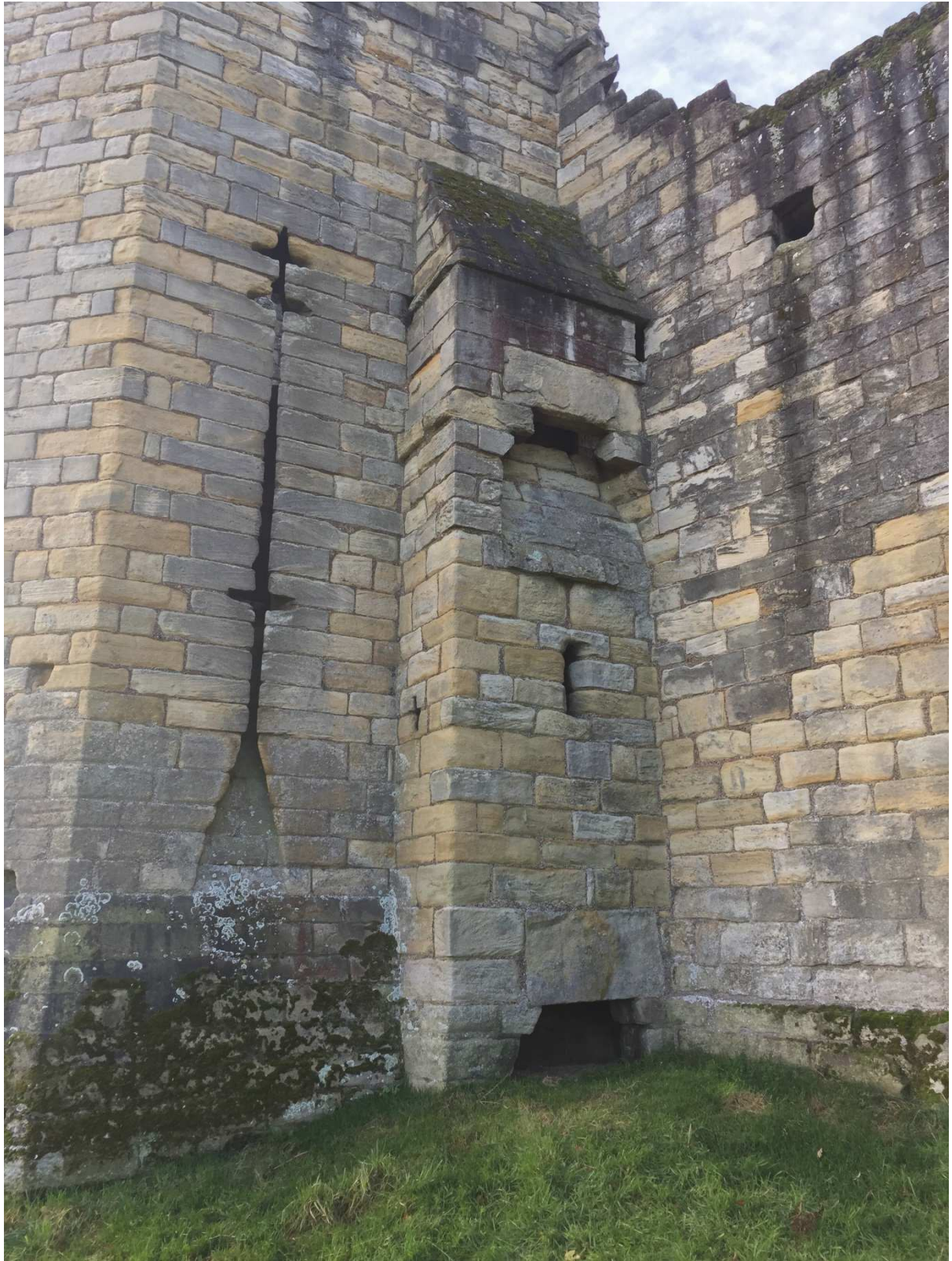
Figure 6. Photograph of latrine chambers adjacent to the Grey Mare's Tail Tower, looking south-west. © William Wyeth
