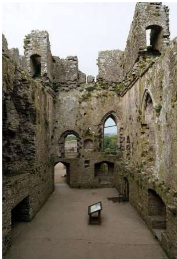
Figure 37: Inner ward: the Great Hall interior, facing WNW. Nb. low, timber first floor (now gone), and ground- and first-floor fireplaces in south wall, to left.
